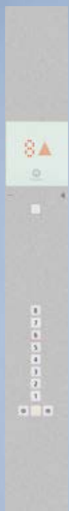
Car operating panel
